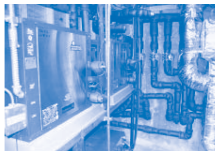
Three of the seven ground-source heat pumps. Black insulated lines go to the ground loops in the 14 borings
