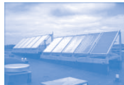
Solar panels on roof send heated fluid to heat water in basement tanks.
