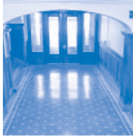
Renovation uncovered this marvelous porcelain floor in the entrance way under multiple layers of flooring.
